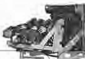
PLB in open position with fuses racked-out
