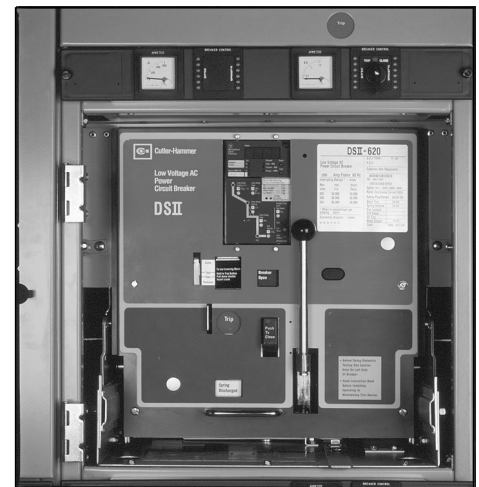
Cell With Breaker
