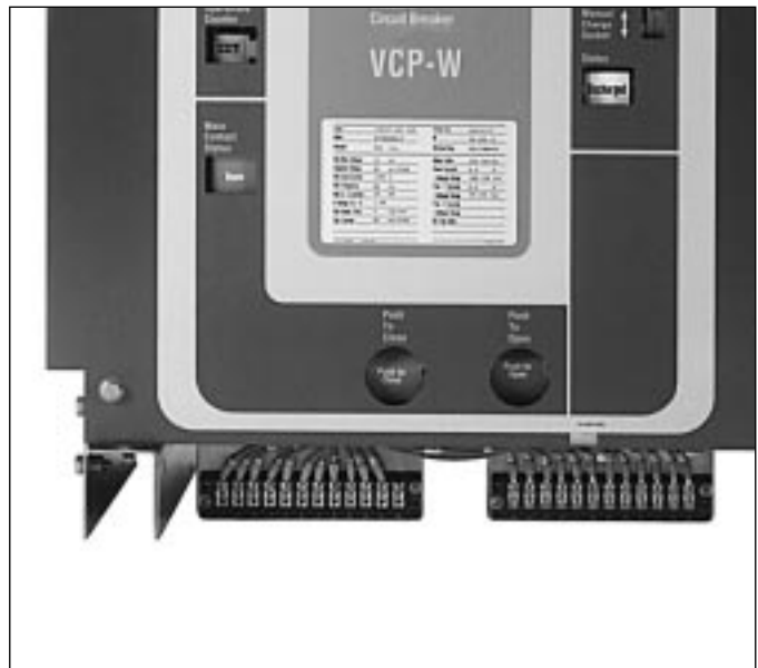
Figure 5-7 Standard Secondary Terminal Blocks Shown Mounted
