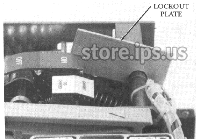
Figure 2. Flag lockout plate installed in breaker.
