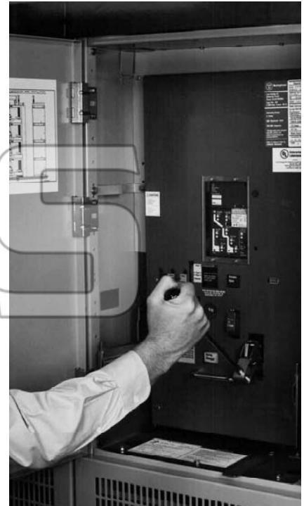
Two-Step Stored-Energy Closing
