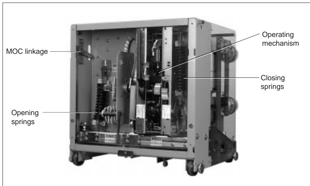
Figure 5: Circuit breaker, right front view without cover
