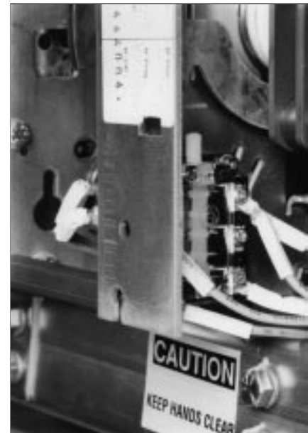
Figure 8: Motor limit switch
